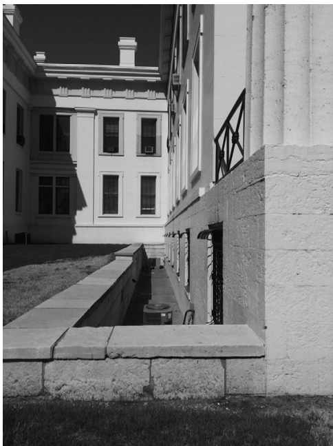
moat condition before
