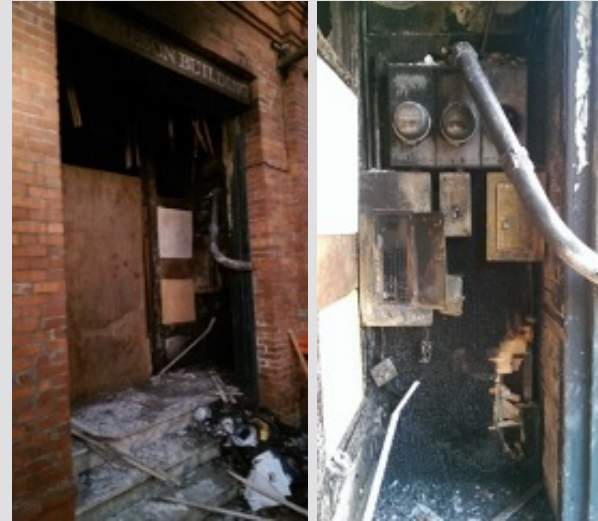
Electrical panel post-fire
