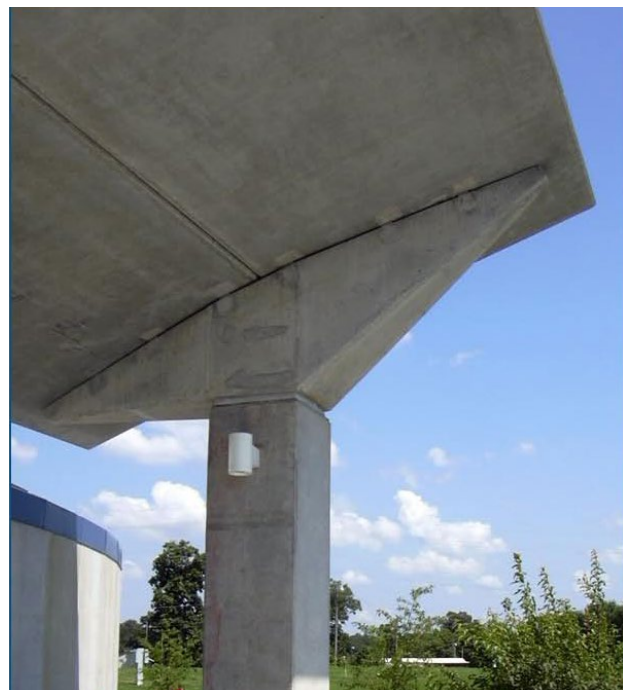
Canopies mounted on concrete piers designed to withstand 250-mph winds provide weather protection
