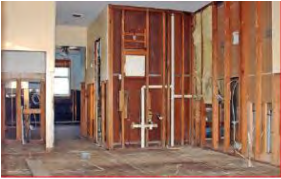
Figure 12-6: As a result of an estimated 0.9-1.2 m (3-4 ft) of flooding, interior walls had to be replaced as well as an exterior door and window. [Source: FEMA]
