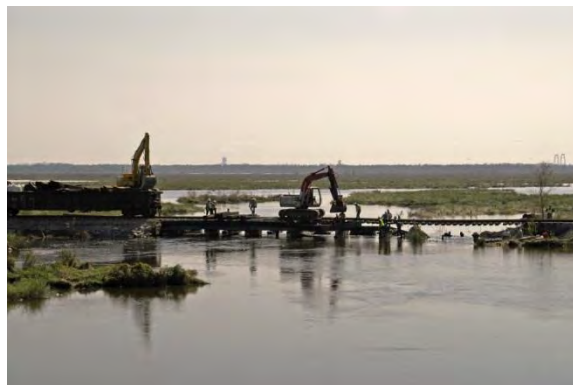
Figure 13-4: A railroad bridge in New Orleans was washed out by flooding during Hurricane Katrina. (Source: Photo by Marvin Nauman [FEMA 2014c])
