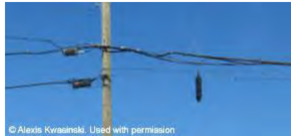
Figure 15-4: Failure of CATV cable due to wind effects
