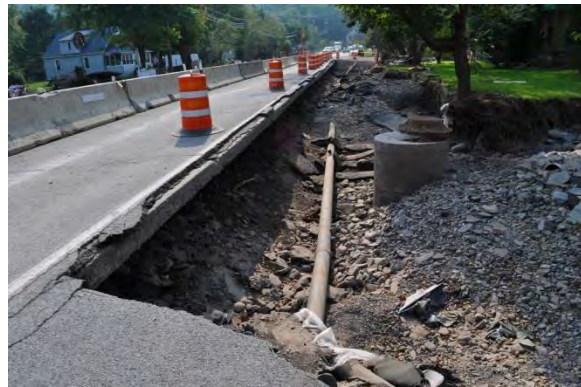
Figure 13-1: Road undercutting in the aftermath of Hurricane Irene (Source: Photo by Elissa Jun [FEMA 2014a])
