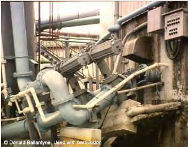
Figure 16-11: Non-pile supported structures failed due to liquefaction in 1995 Kobe Earthquake.
