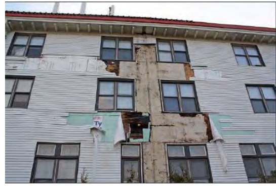
Figure 12-7: Siding loss and minor envelope damage on low-rise building from a wind event [Source: FEMA]
