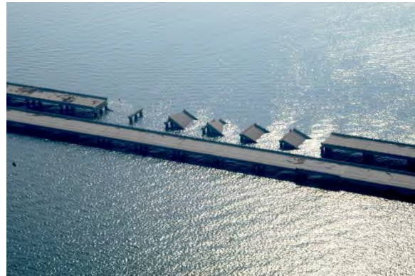
Figure 13-3: Bridge sections knocked off their supports during Hurricane Katrina due to wave action. (Source: Photo by Win Henderson [FEMA 2014d])
