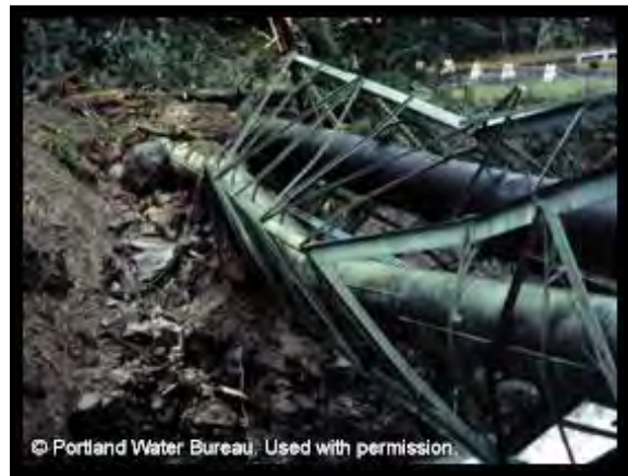
Figure 16-2: Water transmission pipeline bridge damaged by landslide
