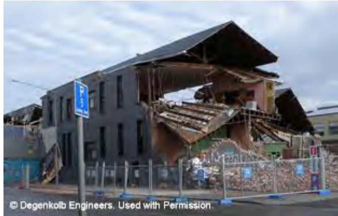
Figure 12-1: Failure of unreinforced masonry wall during an earthquake event
