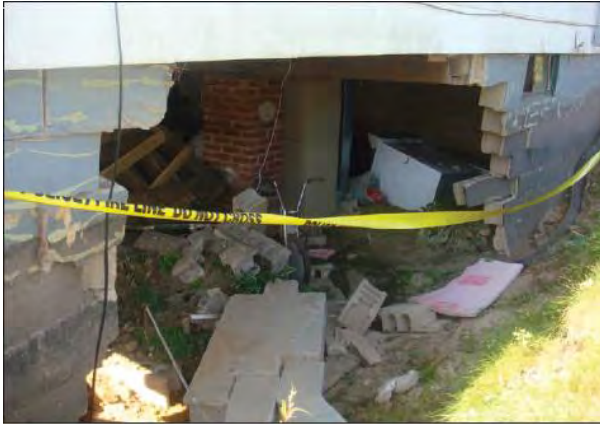
Figure 12-10: Foundation wall collapse due to hydrostatic pressure from floodwaters [Source: FEMA]
