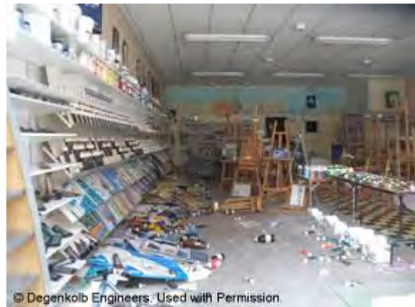
Figure 12-5: Significant nonstructural damage inside structurally stable building after earthquake event
