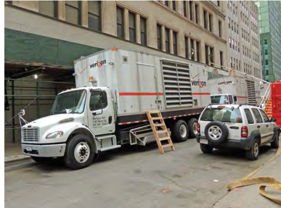
Figure 15-3: Large standby portable power unit used when basement generators failed [Source: FEMA 2013]
