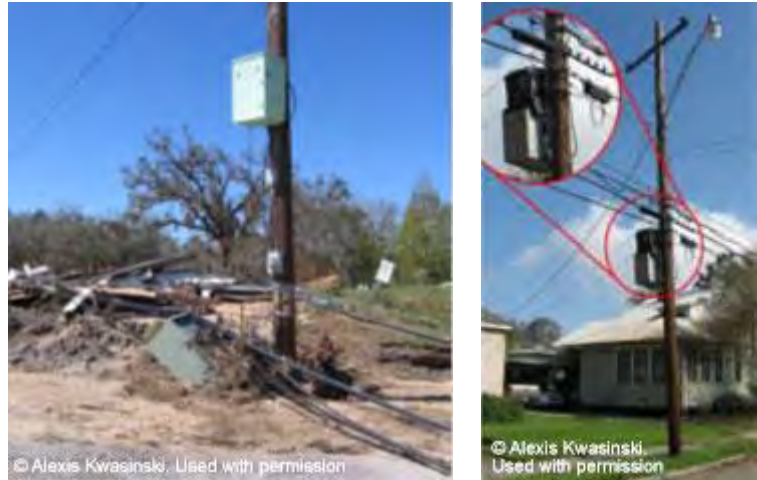
Figure 15-6: Placement of UPS systems is an important consideration for resilience and periodic maintenance.
