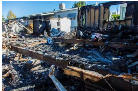
Figure 13-9: Fire damage from broken gas lines [Source: Christopher Mardorf, FEMA 2014]
