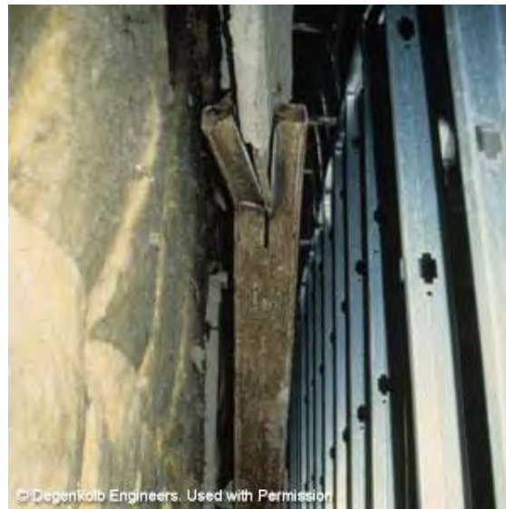
Figure 12-9: Fractured brace connection in a building damaged in an earthquake
