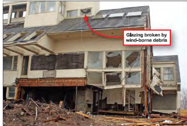
Figure 12-11: Wind and wind-borne debris resulted in considerable damage to glazing on this building. [Source: FEMA]
