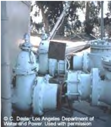
Figure 16-7: Tank moved, severing connecting pipe in 1994 Northridge Earthquake
