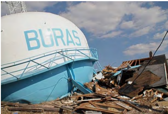
Figure 16-5: Collapsed water tank in Buras, LA near Hurricane Katrina landfall location [Source: FEMA]
