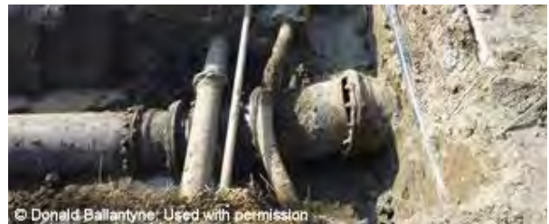
Figure 16-4: Liquefaction caused differential settlement between pile-supported structures and buried pipe during the 2011 Tohoku Earthquake
