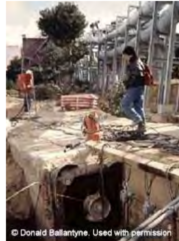
Figure 16-12: Higashinda WWTP Channel offset by liquefaction in 1995 Kobe Earthquake
