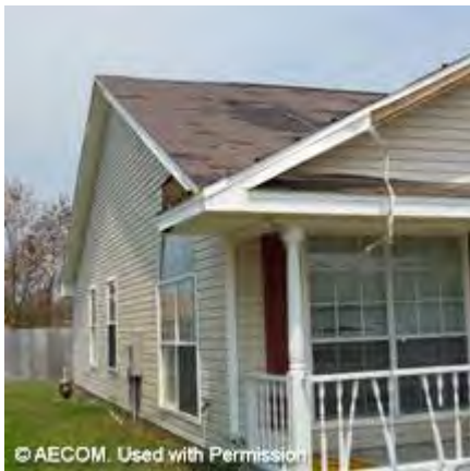
Figure 12-4: Damage to roof covering, vinyl siding and fascia as the result of wind
