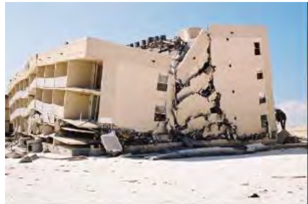
Figure 12-12: Collapse of five-story building due to undermining (from flooding) of shallow foundation [Source: FEMA]
