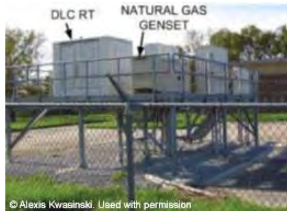
Figure 15-5: Elevated DLC RT with natural gas standby generator installed after Hurricane Katrina
