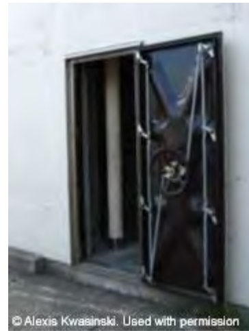
Figure 15-7: Watertight door used on central office in Kamaishi, Japan
