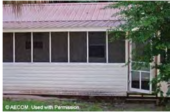
Figure 12-3: Floodwaters reached just under the first floor on this building.
