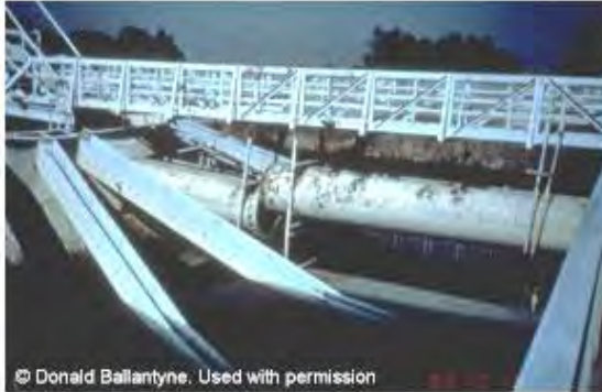
Figure 16-3: Santa Clara Valley Water District, water treatment plant clarifier launders damaged due to sloshing, 1989 Loma Prieta Earthquake
