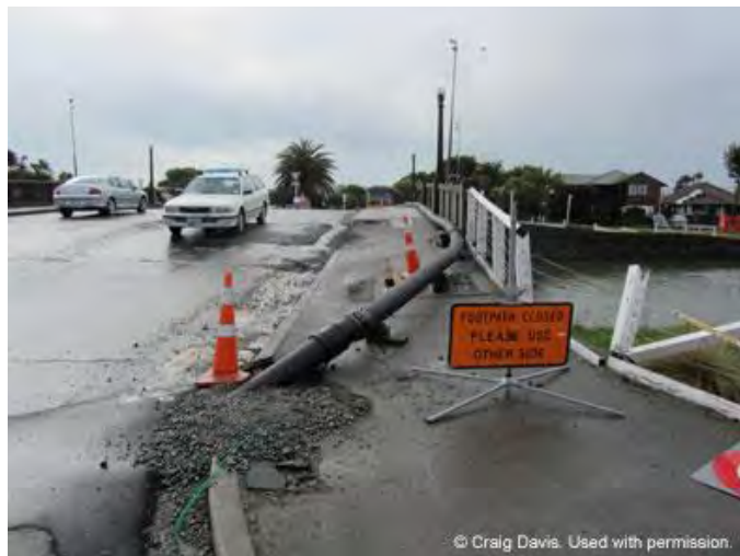
Figure 11-6: Example of infrastructure co-location
