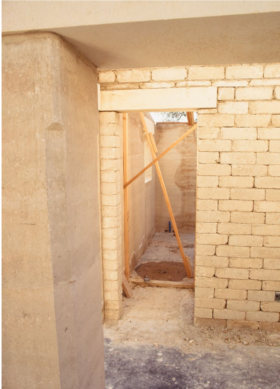
under construction view of limestone lintels over doorways of "caliche" rammed earth walls with corner chamfer (forefront); compressed earth block wall (behind)
