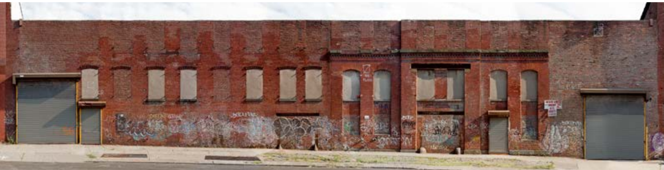
(BEFORE) Exterior prior to restoration with extensive building graffiti
