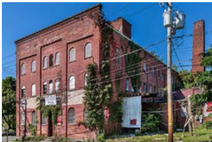
(BEFORE) Exterior state of neglect prior to restoration
