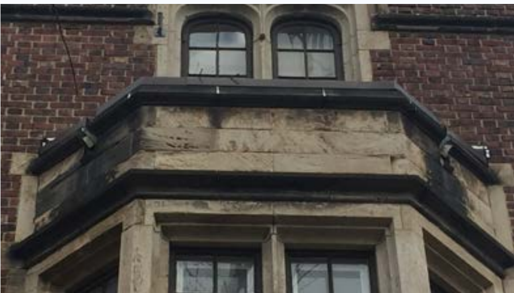
(BEFORE) Exterior stained limestone due to scuppers directing water down face of bay window
